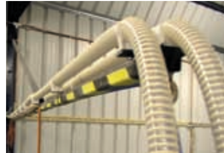
Flexible vacuum ring main provides swinging overhead supply
