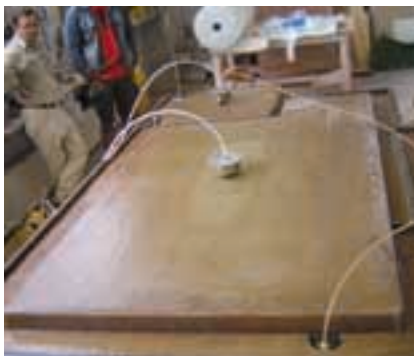
The 15 minute DCPD resin fill approaches the final catchpot
